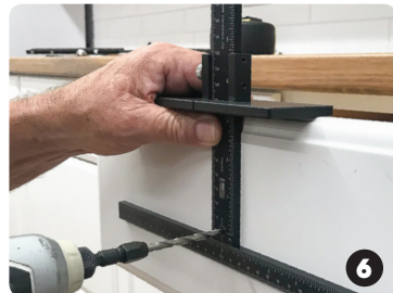
Drill hole using fixed center drill bushing (Large stop reversed for stability)
