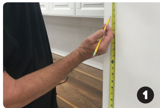
Measure and mark desired location of center hole to be drilled (we are drilling in sets of three)
